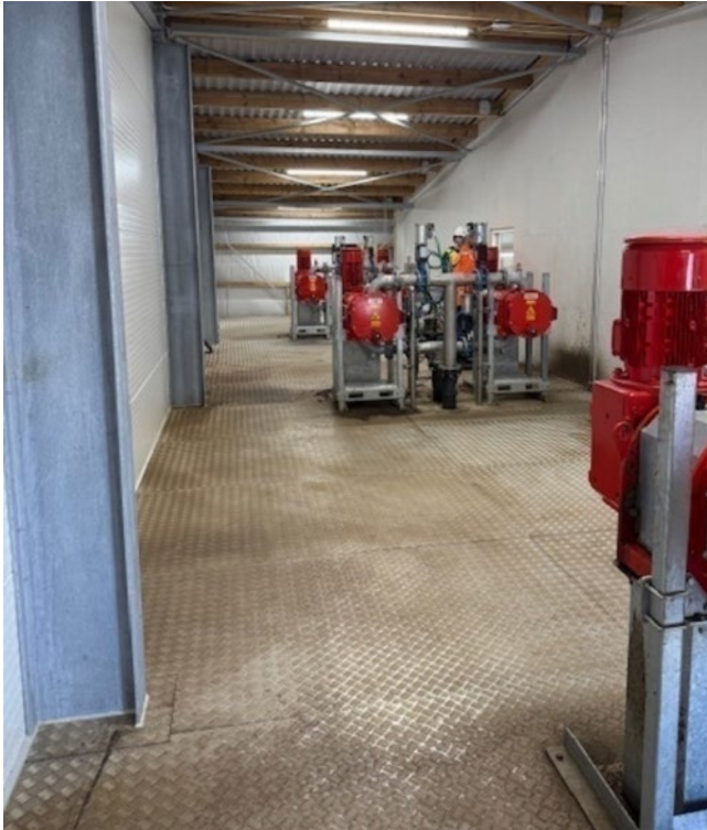
Figure 3-9: Screw Press Separator Units
