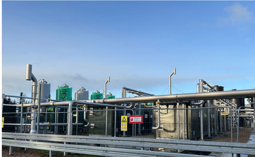
Figure 3-35: CO 2 Liquefaction Plant (Tonder Biogas)
