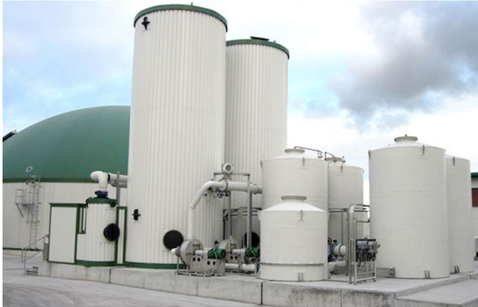
Figure 3-33: Biogas Desulphurisation Plant Source (CSO Group, 2026)
