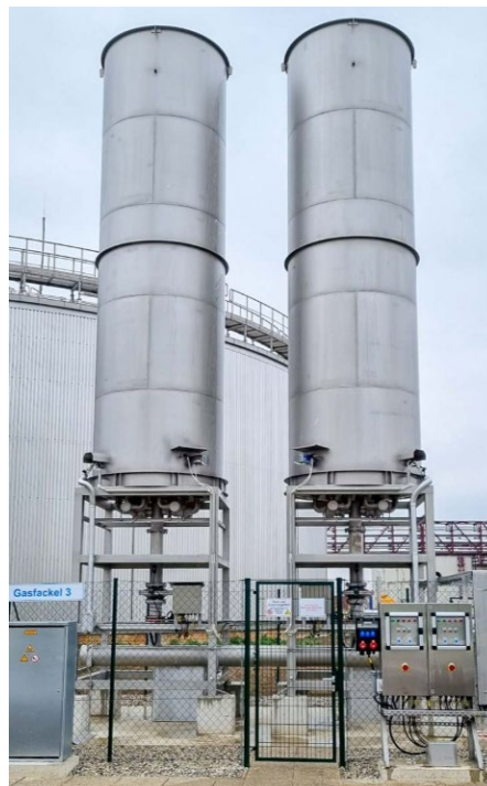
Figure 3-14: Typical Enclosed Flares (Himmel)
